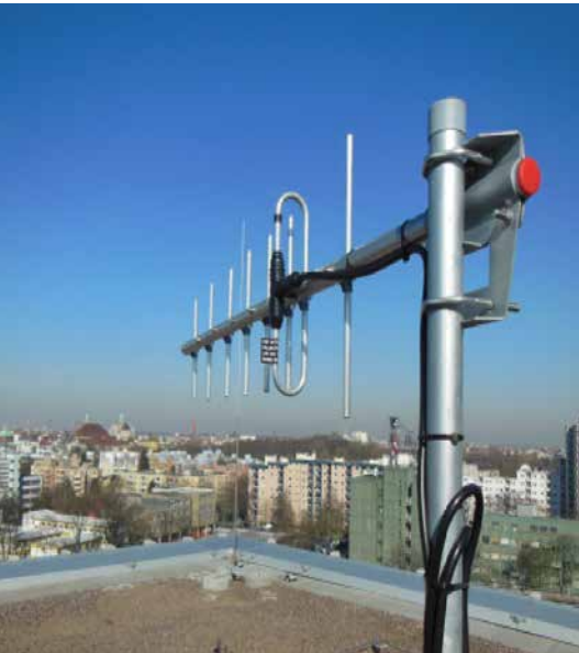
Objektversorgungstechnik. Photo: BDBOS. Indoor radio coverage equipment.
