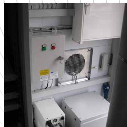
Blick in den Technikraum des Containers. A view into the technical space in the con- tainer.
